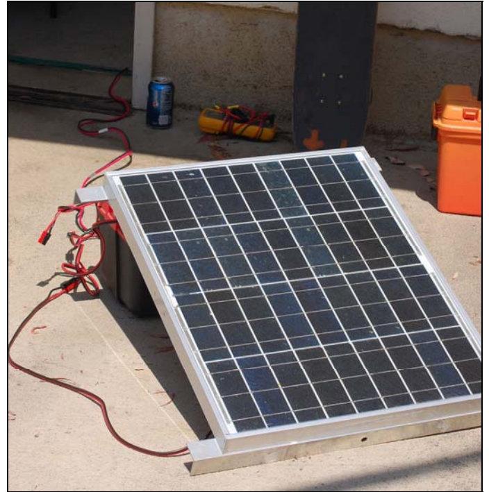
KD6CMO's solar panel, controller and battery outdoors.
