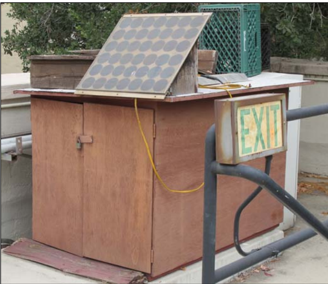
This is where the generator sleeps. Its battery is trickle charged by a solar panel to always be ready for a wake-up call.
